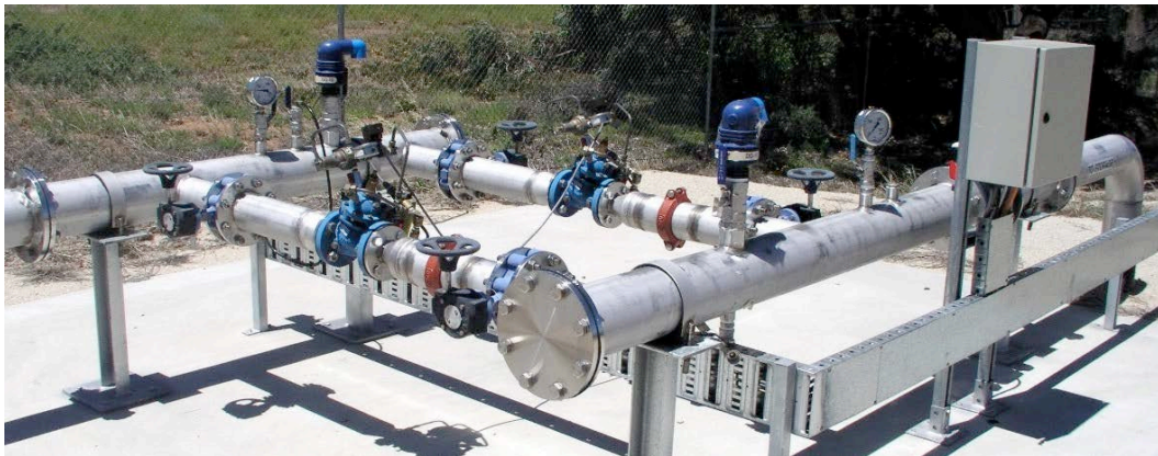
Fig. 6 Wimmera Mallee Pipeline: A typical inlet control valve (ICV) assembly.
