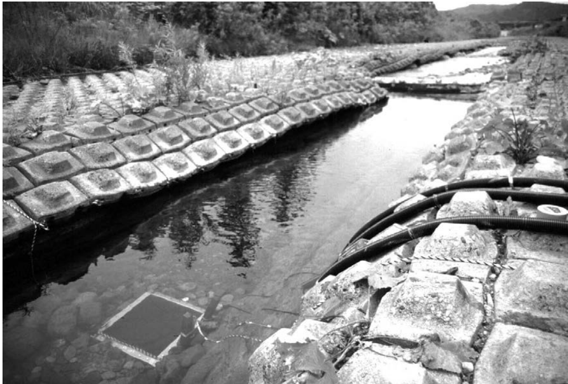
Fig. 2 Condition of the improved channel in July 1997. A pressure-pillow sensor set on the bedrock of the river also can be seen (photo by Y. Kurashige).
