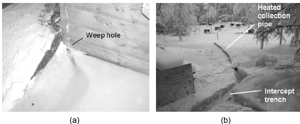
Fig. 3 Emergency corrective action measures: (a) crawl space drainage, and (b) intercept trench.
